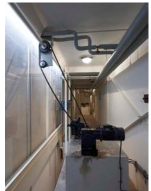
024_VT_Copyright_david_zidlicky_MACHINE ROOM FOR THE WINDOWS.jpg
